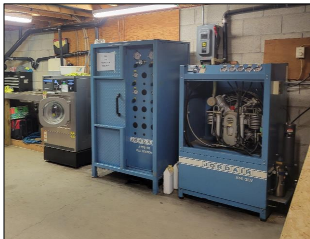
Cascade system, extractor machine, repair area
