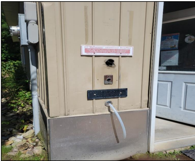
Exterior Water Refill Station
