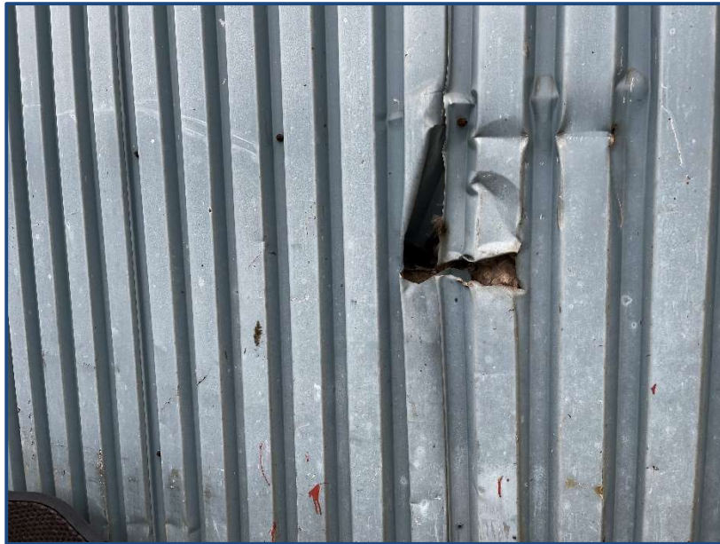
Picture 4: Impact Damage to North Siding of Garage No. 2
