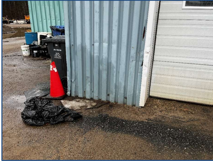
Picture 1: Impact Damage to Siding and Garage Door Frame – Southwest Corner
