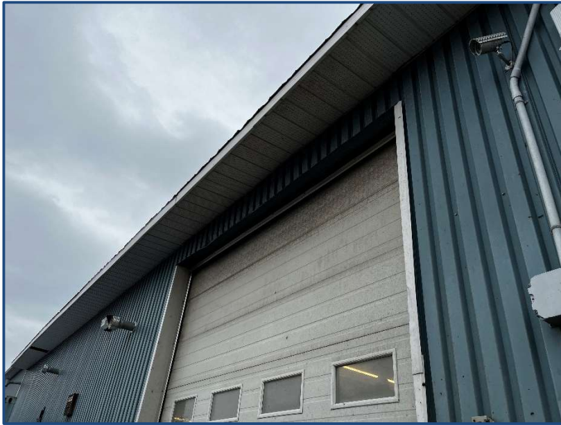
Picture 15: North Garage Door – Damage to Top Left of the Doors Frame
