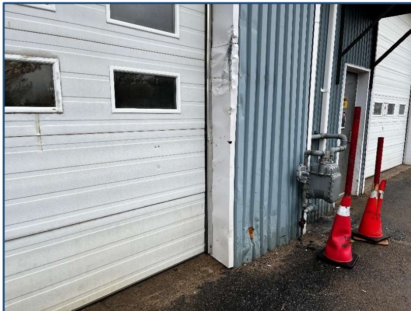
Picture 2: Impact Damage to Garage Door Frame
