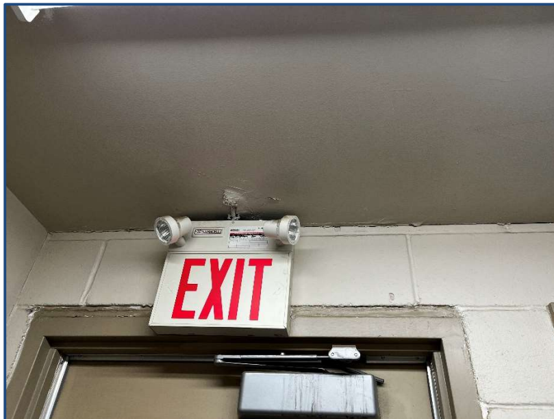
Picture 29: Minor Drywall Cracking and Broken Door Closer
