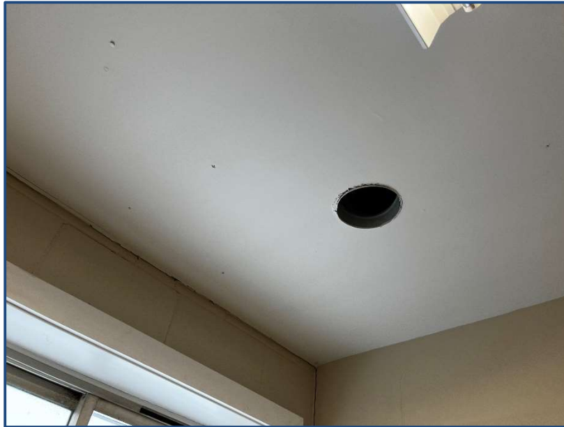
Picture 28: Air Vent Missing Cover – Lunchroom
