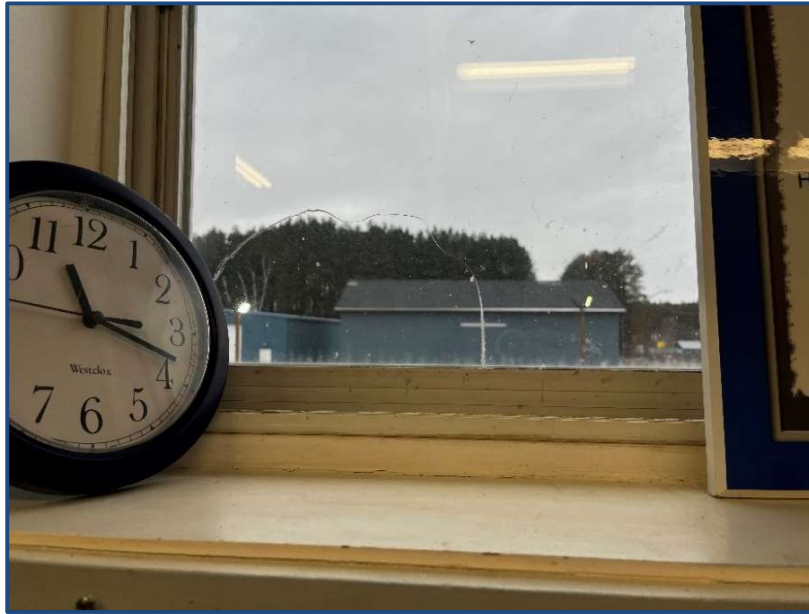
Picture 33: Cracked Window on North Wall of Second Floor Office
