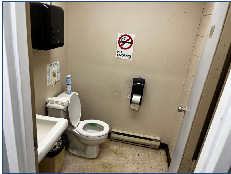
Picture 66: Lack of Toilet Grab Bar Women's Washroom
