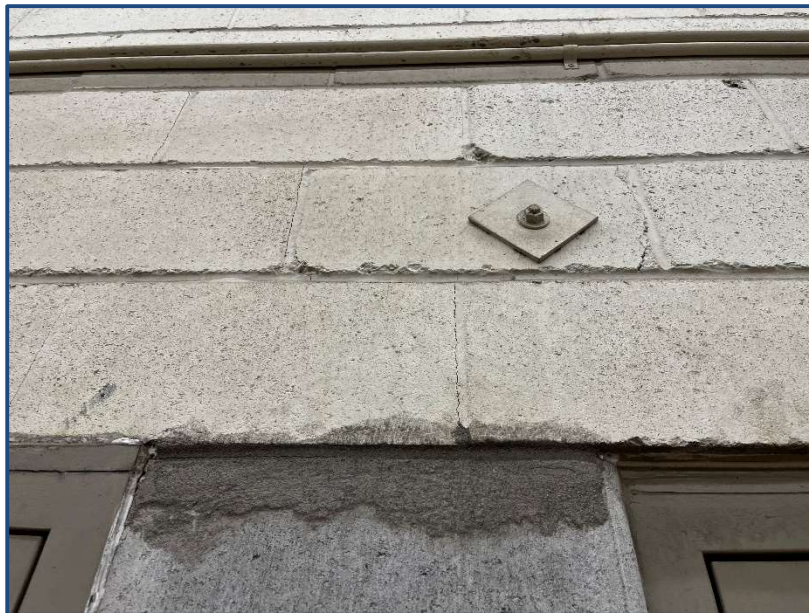
Picture 40: Step Cracking Above the Man Doors on the East Wall
