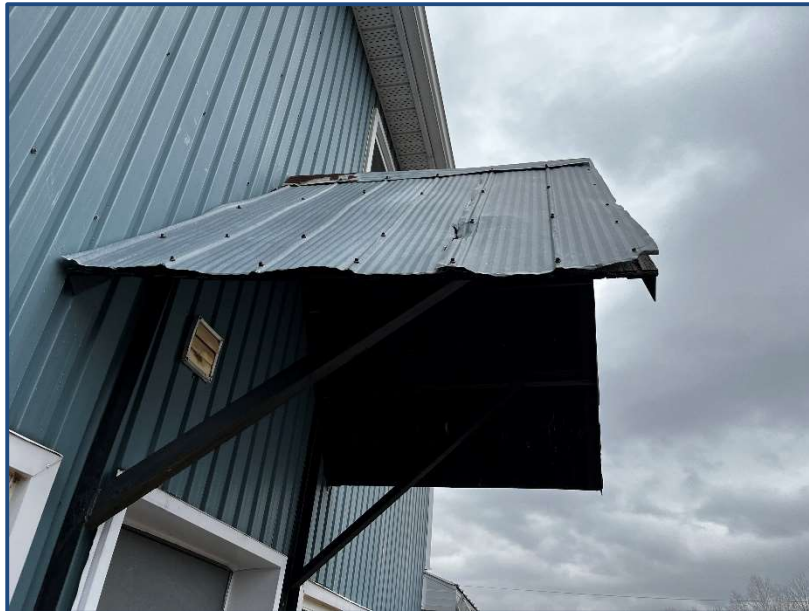
Picture 8: Damaged South Entrance Canopy
