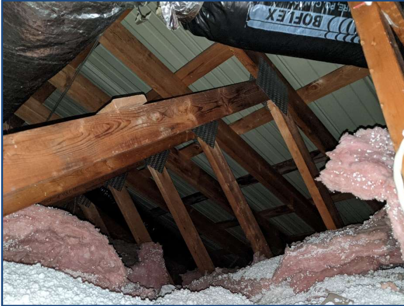
Picture 21: Moisture Staining on First Floor Office Trusses
