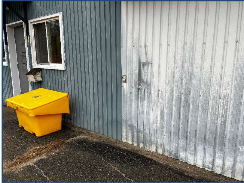
Picture 3: Impact Damage to Siding of First Floor Offices
