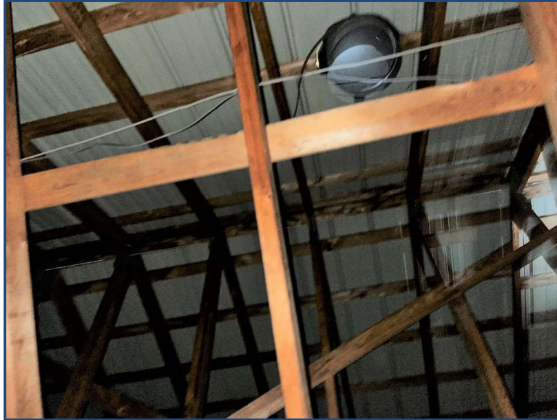
Picture 35: Localized Water Staining in Second Floor Attic
