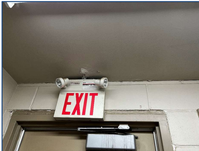
Picture 70: Outdated Emergency Exit Signage – Locker and Lunchroom South Entrance
