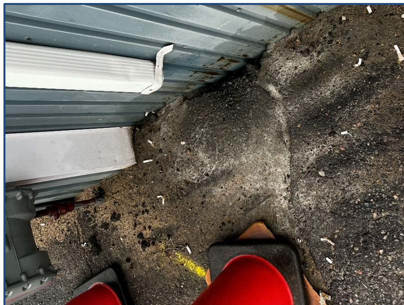
Picture 6: Roof Drain Eroding Asphalt
