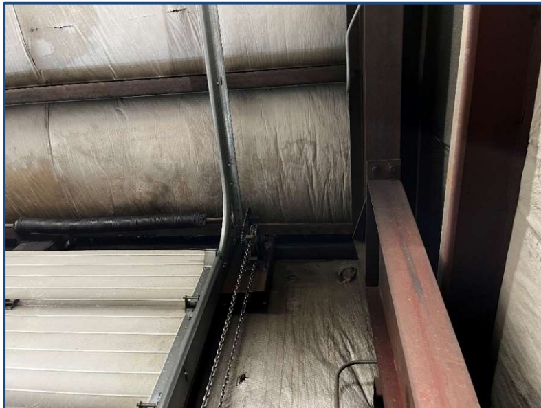
Picture 61: Rotated Steel Beam at Southwest Corner of Huntsville Operations Centre
