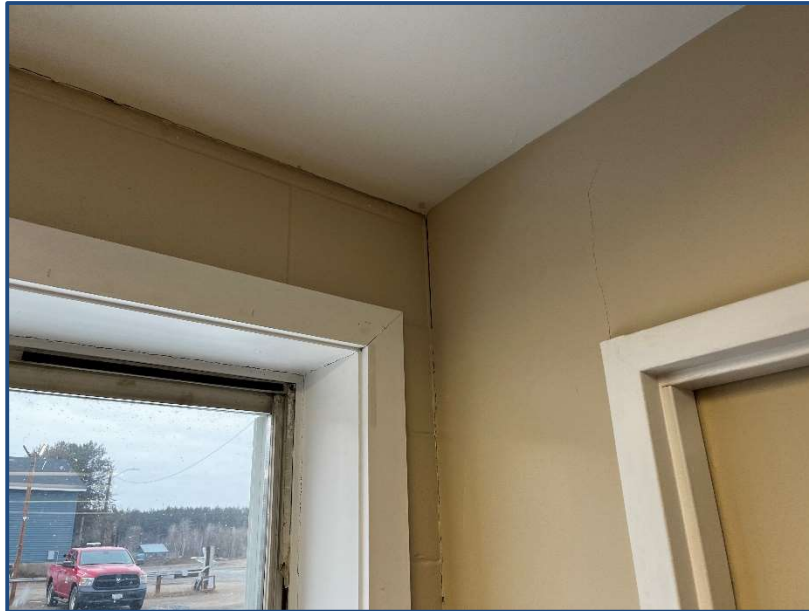
Picture 26: Cracking of Drywall above Interior Door Frame
