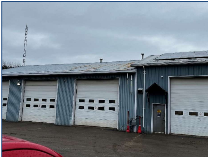
Picture 16: Corroded Metal Roof Panels
