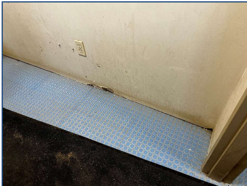
Picture 27: Water Damage at Drywall Base – South Man Door Entrance
