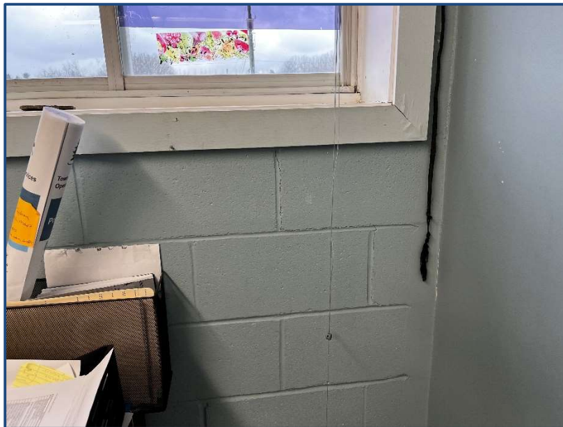
Picture 34: Narrow Step Cracking in Concrete Block Wall – East Wall
