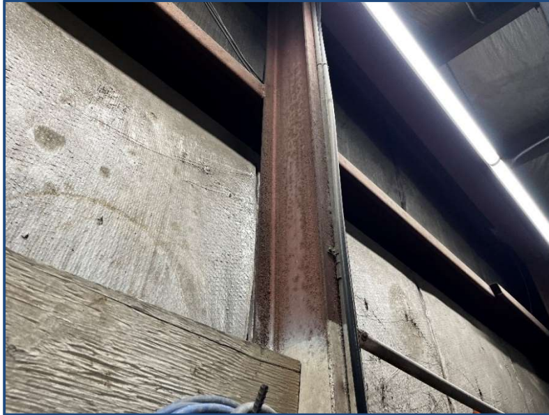
Picture 60: Light Corrosion of West Wall Column
