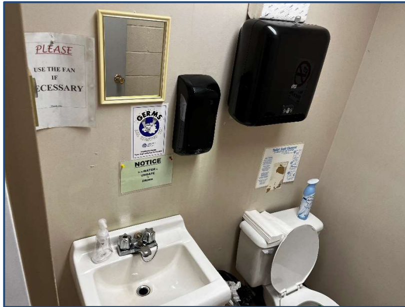
Picture 65: Inaccessible Soap and Paper Towel Dispensers in Women's Washroom
