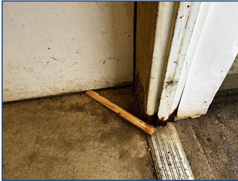
Picture 45: Corroded Steel Door Frame of North Man Door
