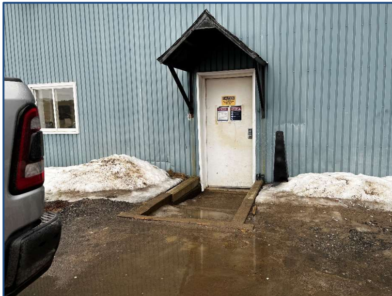
Picture 14: North Garage Side Entrance Below Grade – Watering Pooling at Entrance
