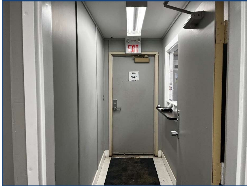
Picture 69: Outdated Emergency Exit Signage – Huntsville Operation Centre Main Entrance
