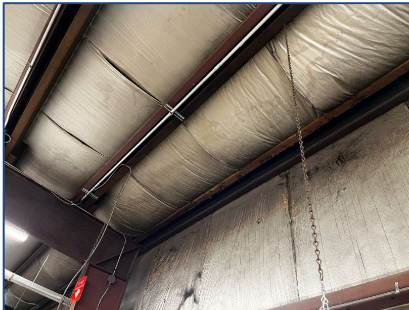
Picture 58: Rotting Timber 1x4 Plank and Sagging Insulation
