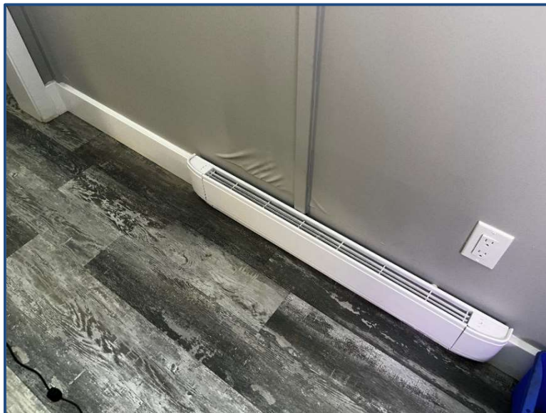
Picture 18: Paint Bubbling above Heater
