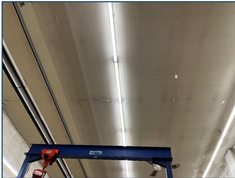
Picture 46: Water Damaged Drywall Ceiling
