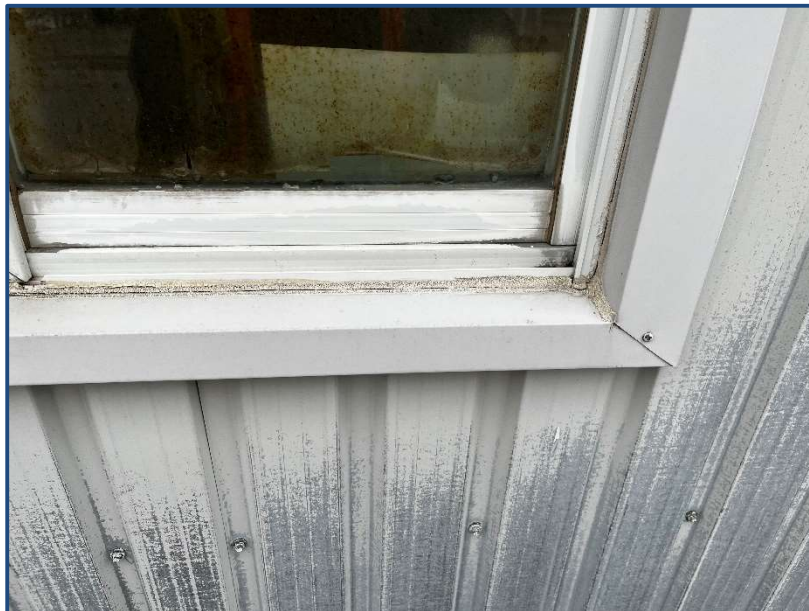
Picture 12: Failed and Cracked Caulking on First Floor Offices Windows
