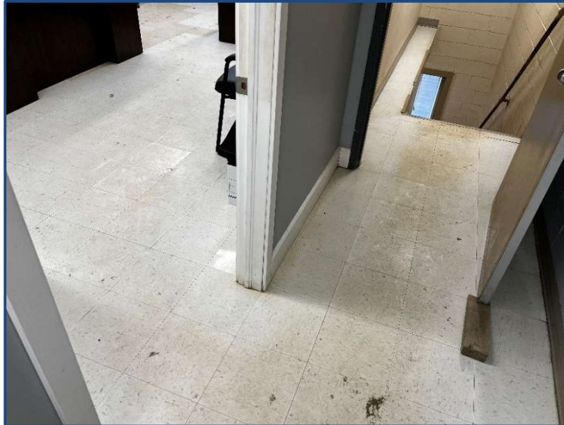
Picture 31: Wear of Vinyl Floor Tiles
