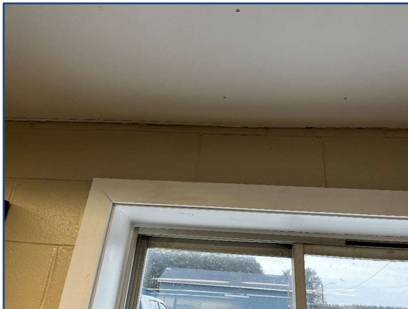
Picture 25: Step Cracking in North Concrete Block Wall
