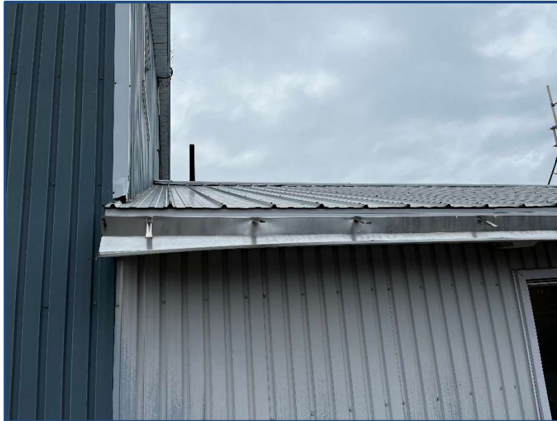
Picture 11: Damaged Eavestrough on First Floor Offices
