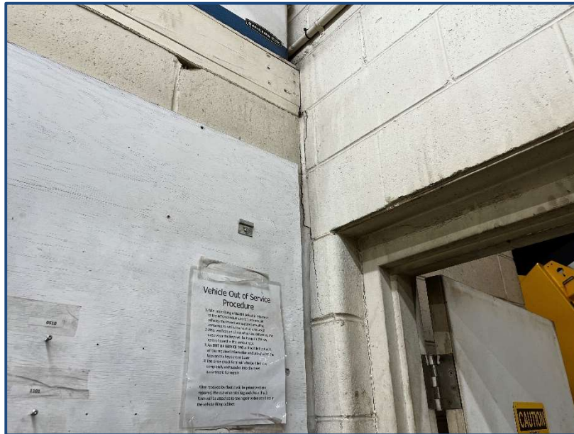
Picture 36: Cracking in Block Wall between Garage No. 1 and No. 2
