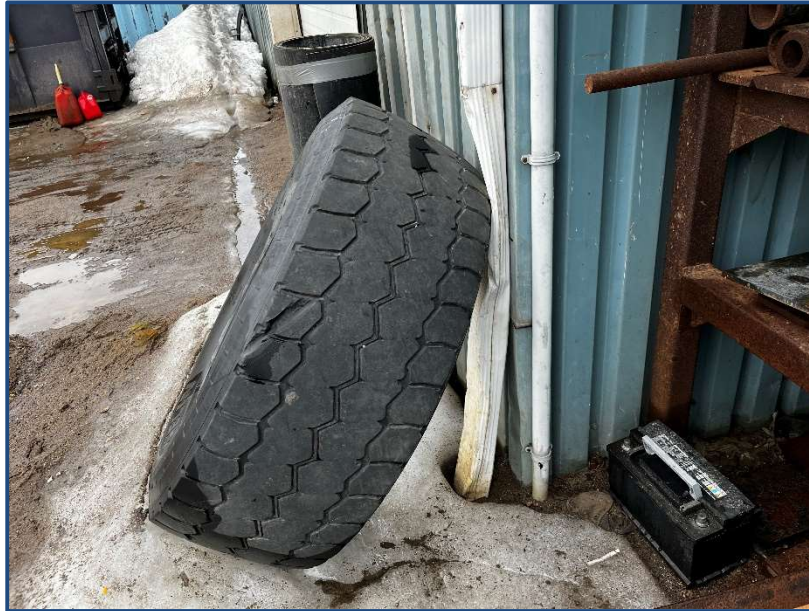
Picture 7: Northwest Crushed Eavestrough Downspout
