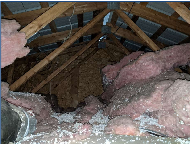
Picture 22: Poor Insulation Spread in First Floor Office Attic
