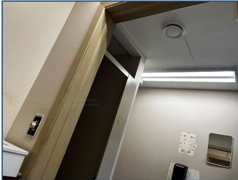
Picture 17: Crack in Men's Washroom Ceiling Paint
